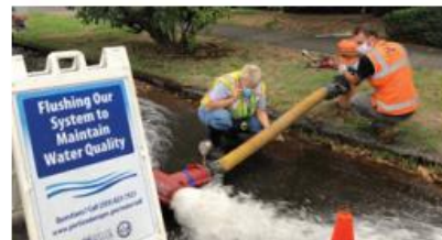
Crews continued flushing water mains in east Portland, cleaning out and maintaining water quality in close to 200 miles of water main.
